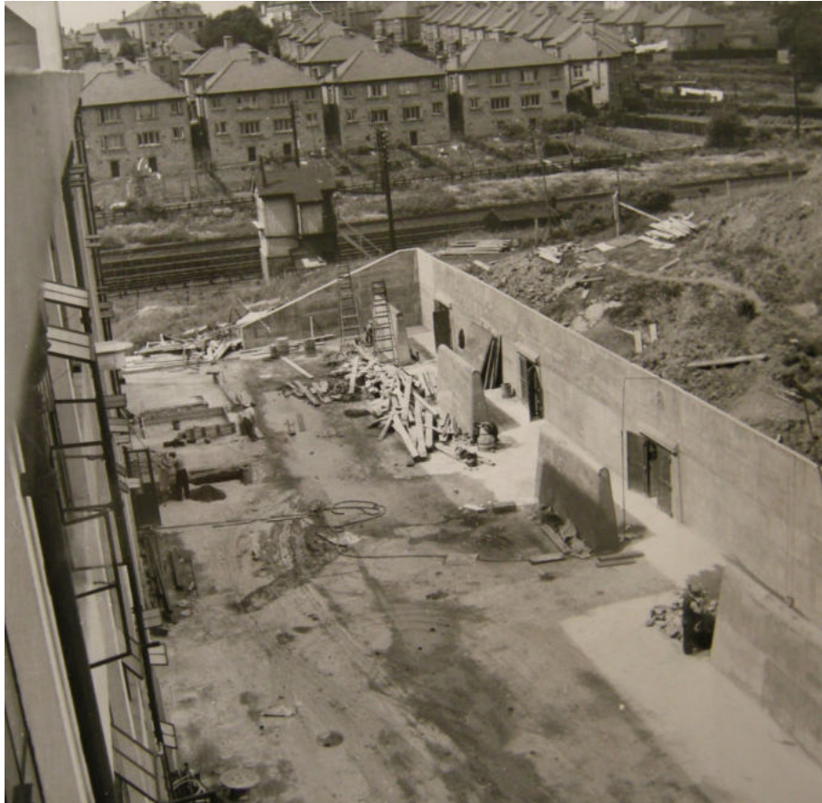
Plate 5: Showing rear of Building 4, the trackside signal box and air raid shelters 1 to 3 under construction (Barnet Library & Local History Centre, 1939)
